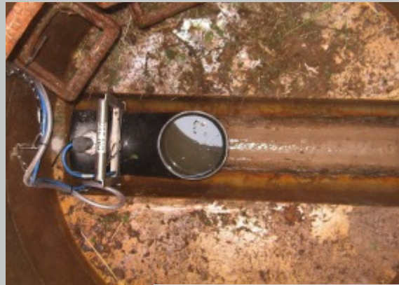
Temporarily installed flowmeter
