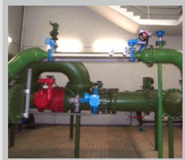
Nighttime supply measurement point in bypass pipeline
