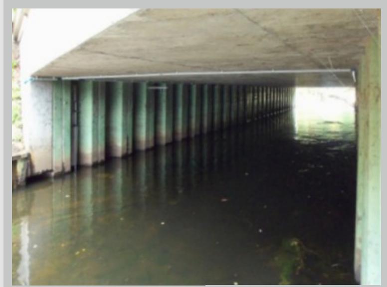
Mounting situation below bridge
