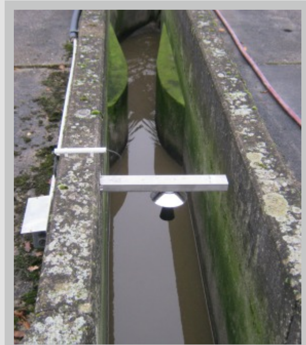
Venturi flume measurement in outlet
