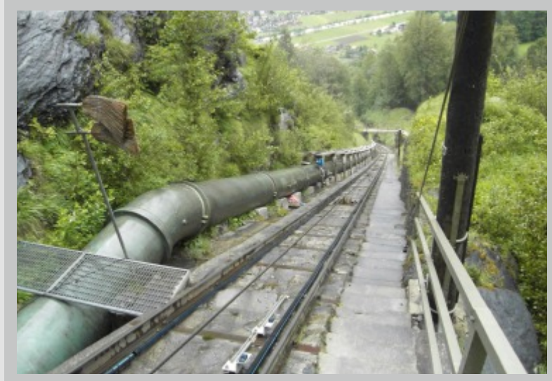
Pipeline down to valley downstream of turbine
