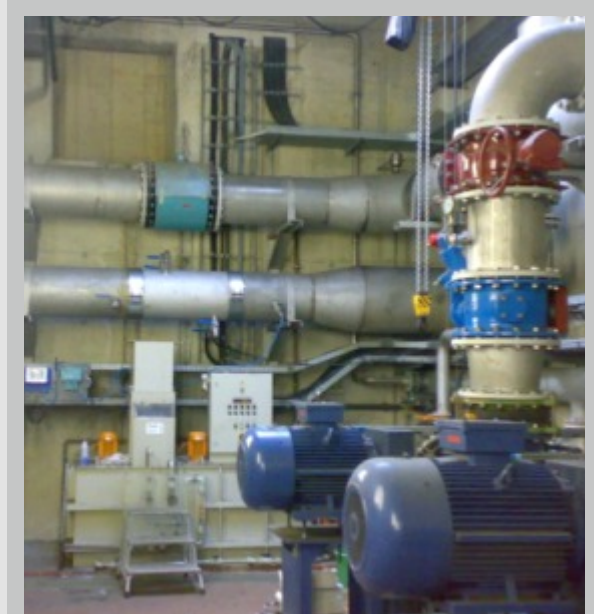
Pump room with discharge line on rear wall
