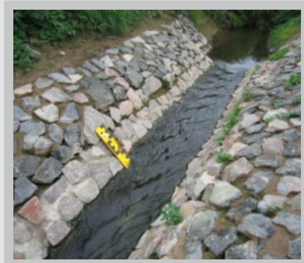
Measurement point with gauge staff
