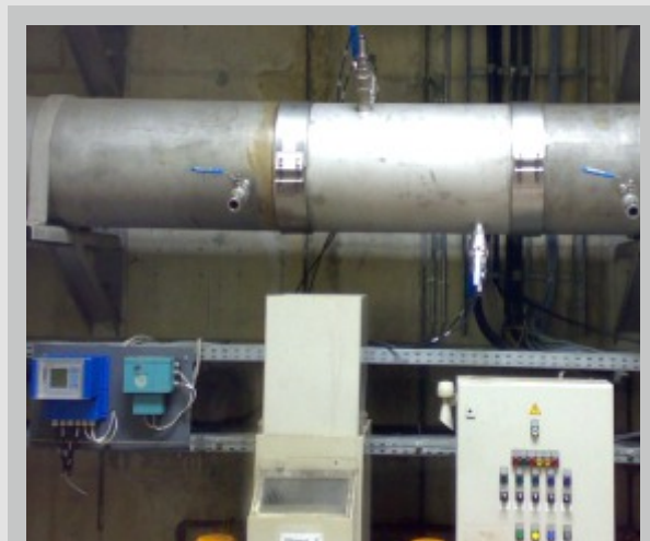
Sensors installed in pipe line
