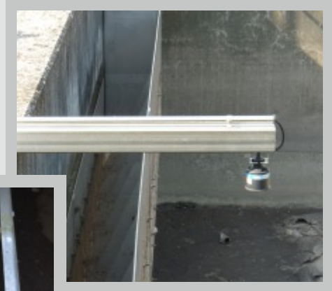
Tank with installed level sensor and data logger
