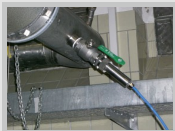
Measurement place with installed sensor
