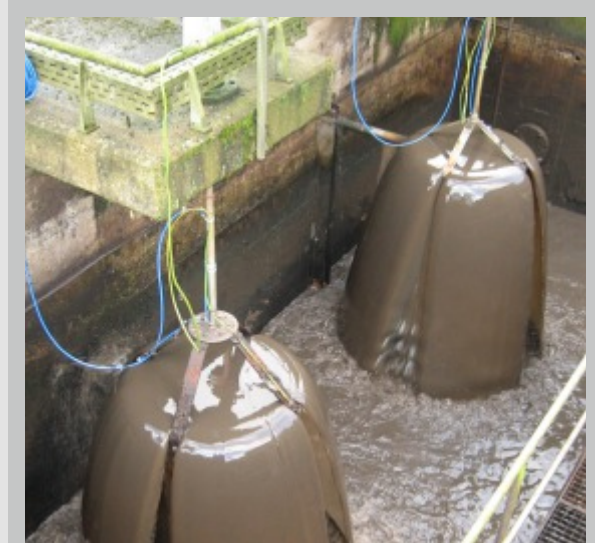
Telescopic pipe in operation
