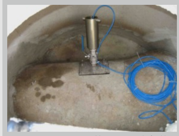
Measurement shaft with extraction tool installed
