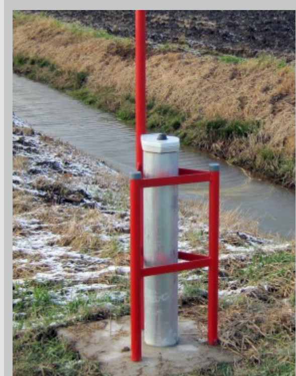
Measuring tube with mast cap and dome antenna
