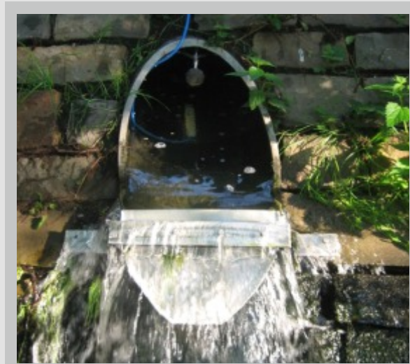
Discharge pipe with impoundage shield
