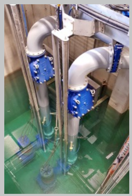
Shaft with immersed pumps and measurement systems
