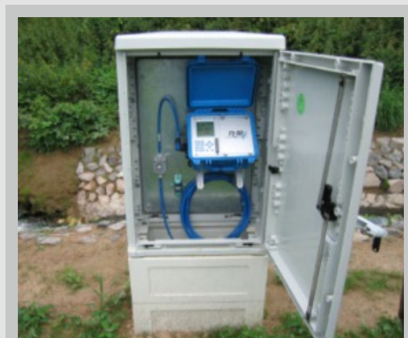
Open control cabinet with transmitter
